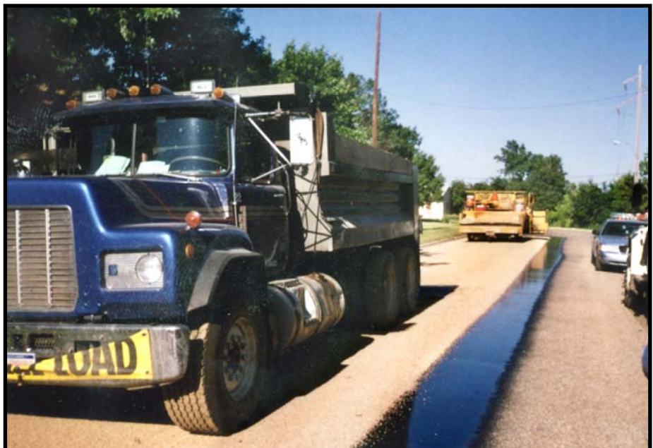
Photo 3 – View from the middle of the roadway showing the work area, with the dump truck unhooked from the rear of the rock-chip spreading machine.
